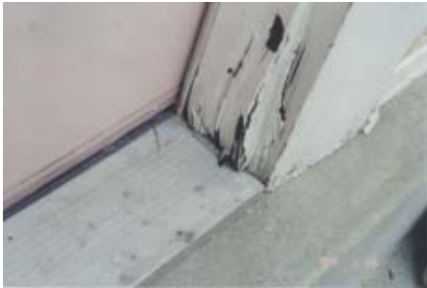
Figure 26 Rot at the bottom of a door frame in a 1990s sample house.
