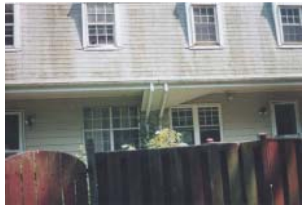
Figure 33 Broken window pane on second-story window.
