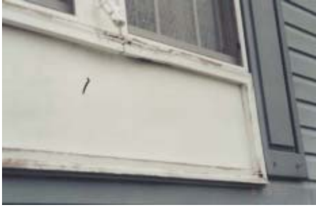
Figure 30 Rot in wood trim associated with poor detailing (i.e., lack of cap flashing) and maintenance in a 1990s sample home.
