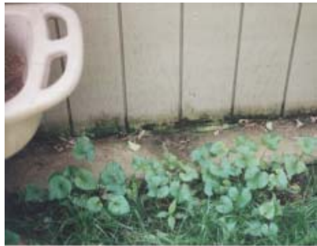
Figure 29 Rot at the bottom of wood panel siding (insufficient ground clearance) in a 1970s sample home.
