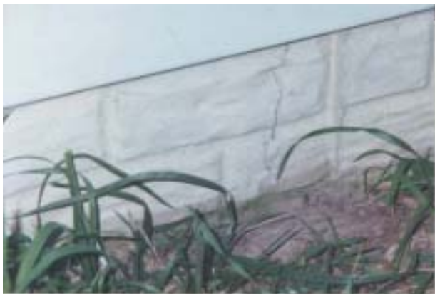
Figure 24 A typical small crack found in a concrete foundation wall.
