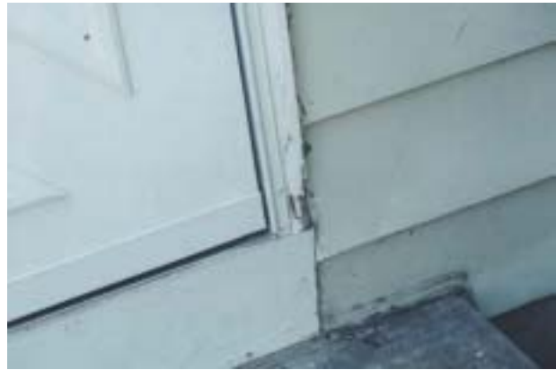
Figure 27 Rot at the bottom of a door frame and trim in a 1970s sample house.
