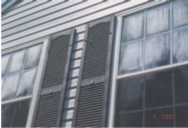
Figure 34 Condensation inside double-pane windows.
