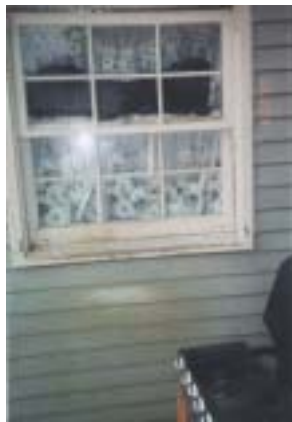
Figure 32 Abnormal wear and tear on a wood window as an apparent result of pet scratching.
